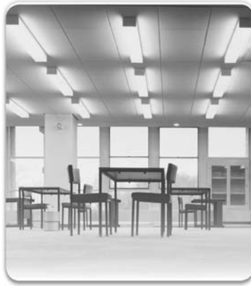
Linear Fluorescent Ballasts
